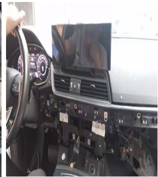
把我司配的专用线材安装好并测试好功能后再复原安装好/Install and test the special cables provided by our company before reinstalling and installing them
