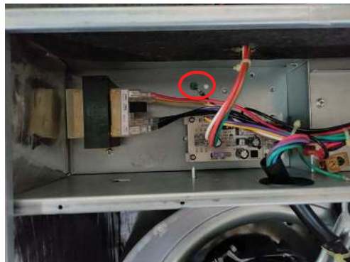
Fig. 7 – Ground to Green Screw (red circle)
