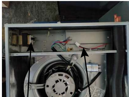
Transformer Power Supply Wire
