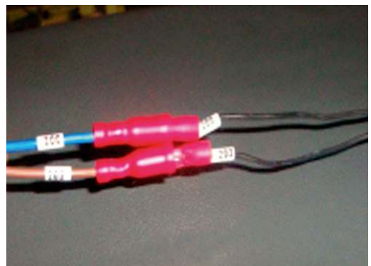
Picture 12 (end switch connection)
