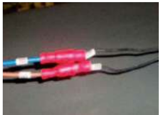
Picture 12 (end switch connection)
