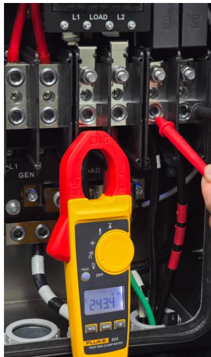
Voltage Check with Multimeter
