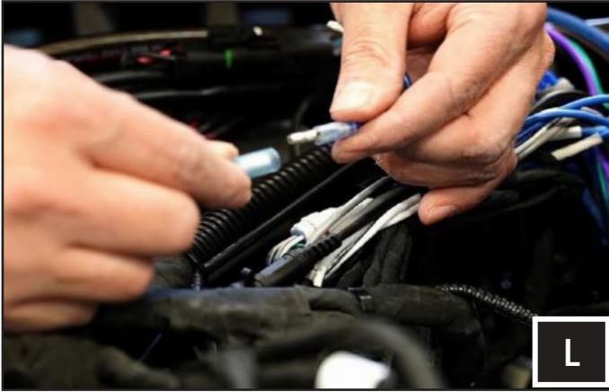
L. Plug in the amplifier's turn-on bullet connectors to the turn-on delay module output wire. See page 6 for reference.
