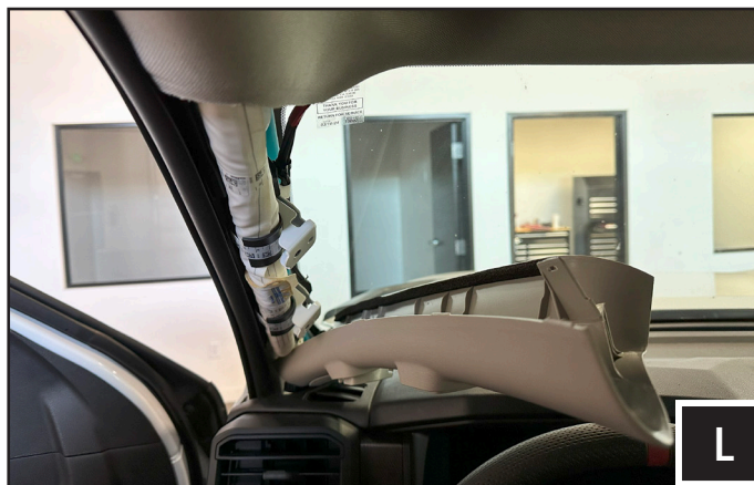
L. Run the ALPHA12 controller cable along the headliner towards the driver side A pillar and down to the firewall. Use the supplied 6 foot controller extension cable and fish through the firewall grommet to the ALPHA12 brain mount location.
