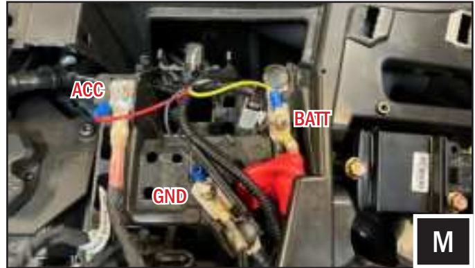
L. Run the BATT, GND and ACC wires of the Power Input Harness (B-H3413) to the factory busbar (top center of dashboard) and screw in the ring terminals to the busbar.
