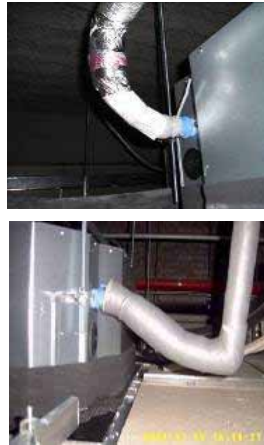
Sample of Bad Installation
