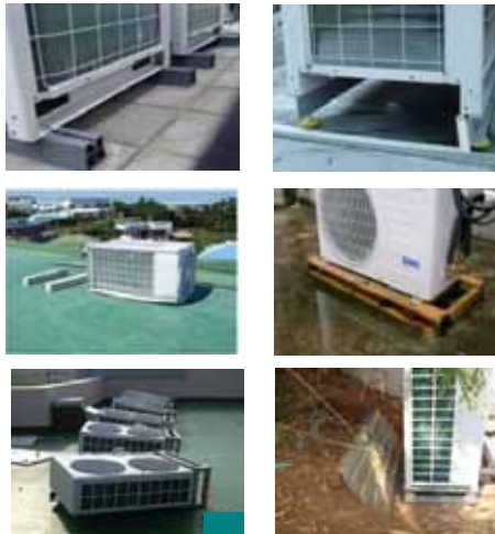
Sample of Bad Installation
